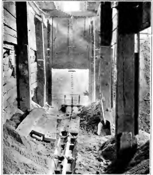
FIG. 1. CLAY SHED SHOWING SCRAPER CONVEYER
